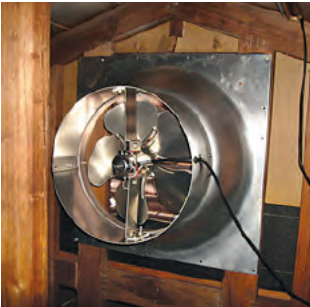
gable mounted fan (view from inside attic)
